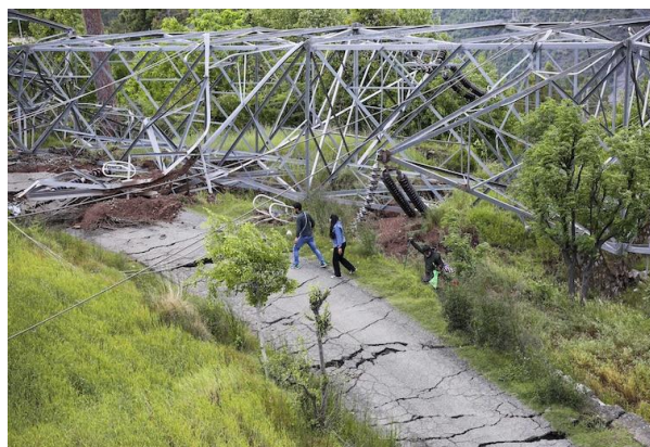
Damaged Electric transmission Tower Source: Media
