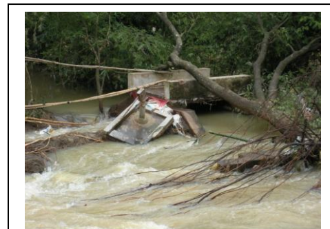
Photo showing damaged handpump at East Chilka village
