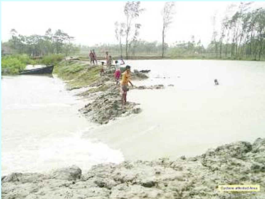
Damaged embankments leading to flooding.
